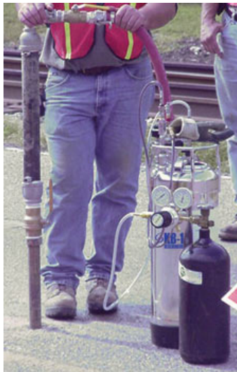
At a site in Indiana, a worker injects the bacteria from steel containers into a pipe that goes underground. The smaller vessel is full of gas that helps push the bacteria down.
